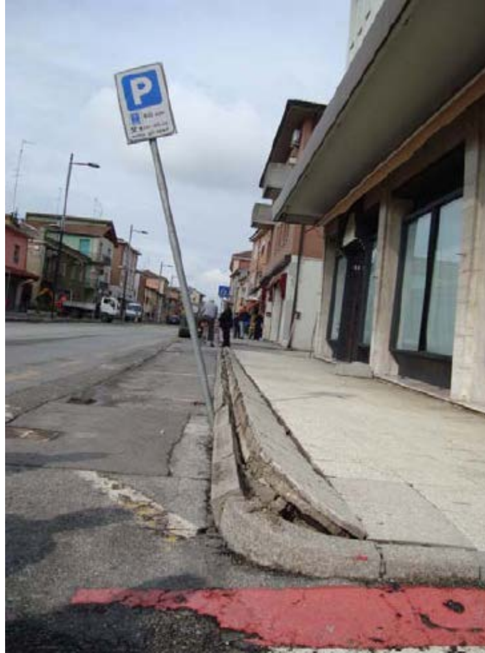
Mirabello, uplift of the floor of the sidewalk courtesy of Florence University
