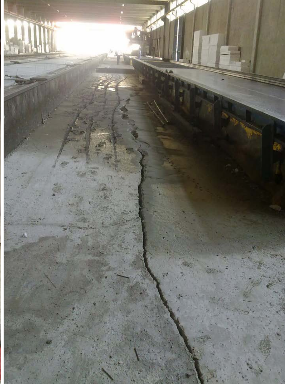
Mirabello, crack in the industrial zone courtesy of Florence University
