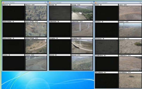
Video-wall at the Command Center, with information from 13 cameras
