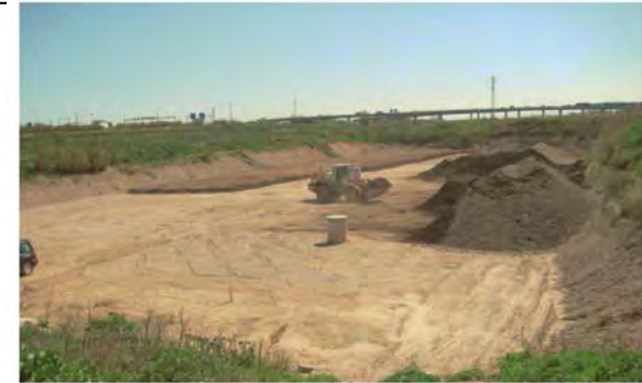
Fig. 1.2: Construction of pilot infiltration basins at Sant Vicenç del Horts near Barcelona.
