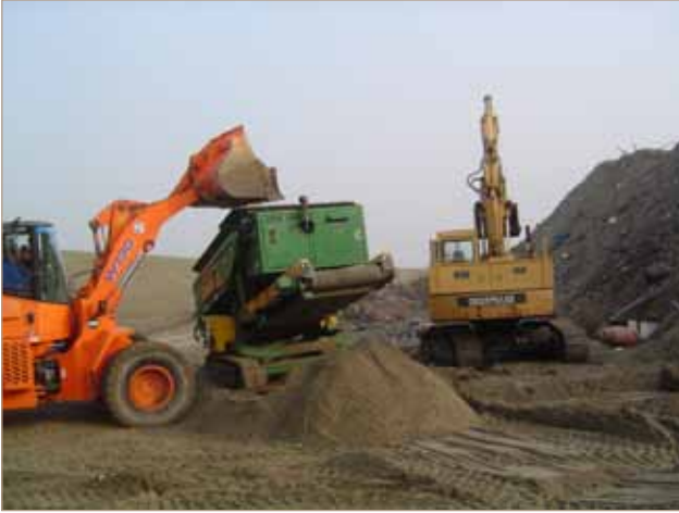
figure 12 Screening the storage area
