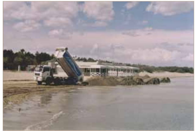
figure 25 Beach nourishment by means of sand from land-based quarries undoubtedly is the solution with the heaviest environmental impact
